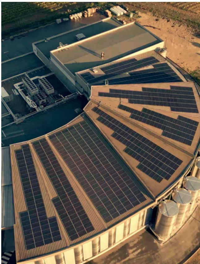
▶ Citizen photovoltaic power plant at the Héraclès winery in Codognan (30) ©ACCTE
